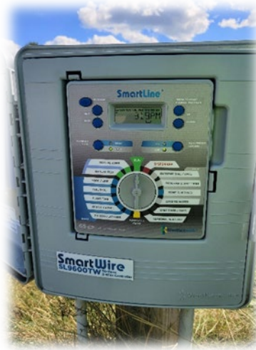
Controller on north side of M-20
