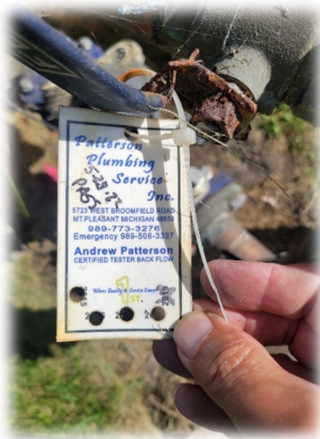
Backflow testing tag
