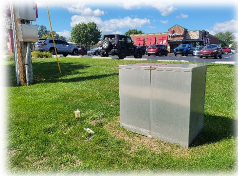
Tap on the north side of M-20
