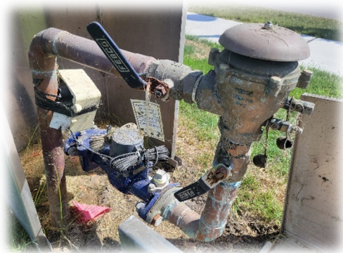
Typical condition of each tap.
