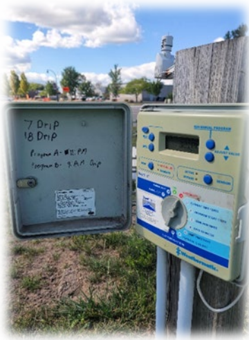
Controller on south side of M-20
